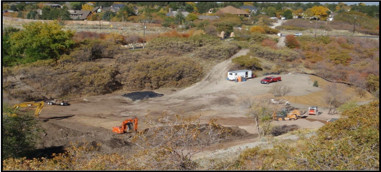
Crews work to remove lead and arsenic contaminated soils in Operable Unit 2, near Little Cottonwood Canyon.
